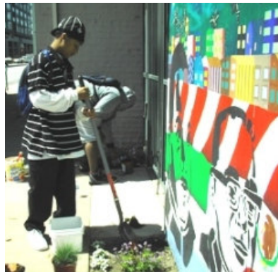
Randy Smith & Marcus Welch carefully work around the sprinklers to add new ornamental grasses.
